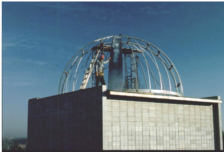
The first panel of skin being installed on the structure of the dome in 1981
